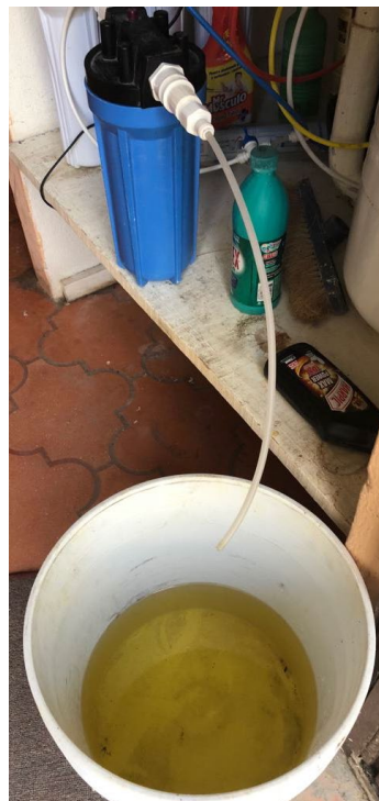
Figure 6.2.3.3 – SPT RO flush yellow outlet water
