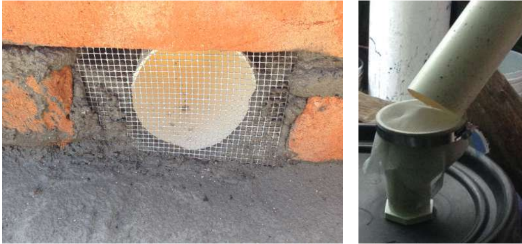
Figure 6.1 — Various leaf filters: (a) an example of a leaf filter installed on the inlet to the gutter system from the roof and (b) the inlet to the first flush.
