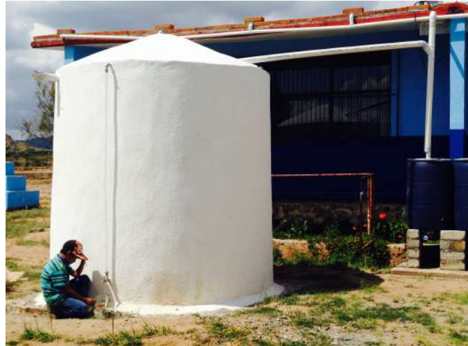
Figure 3.7 — 12,000 liter ferrocement rainwater harvesting cistern, with a 200 liter first flush system and PVC connections to a cement roof.
