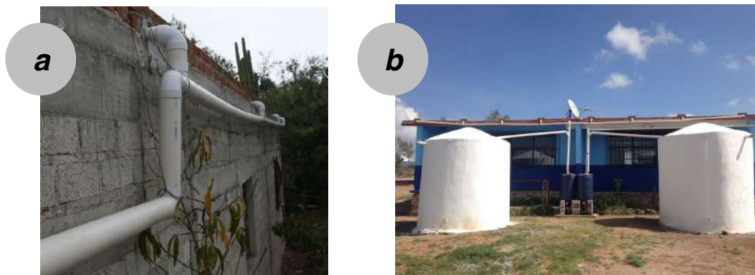
Figure 4.3 — (a) The piping system is connected to four pieces of 2" PVC that carry the water off the roof. The piping is held in place by a double layer of cemented brick. In (b), one concrete flat roof is connected to two cisterns.
