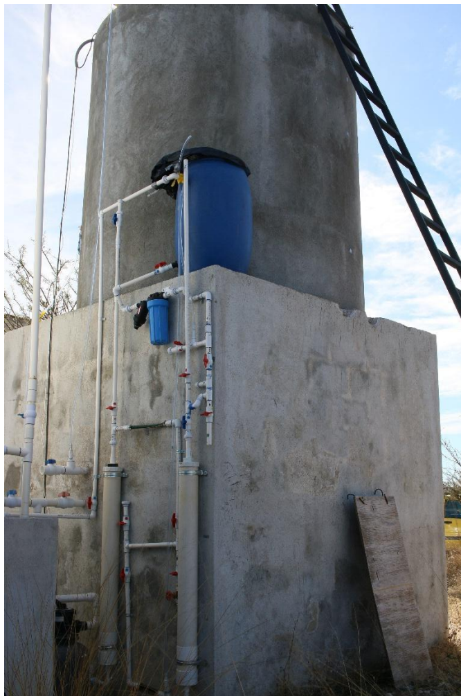
Figure 1: Pilot System for Arsenic Removal
